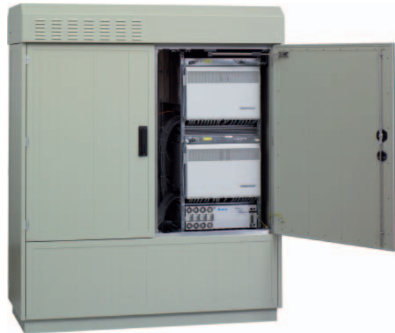
Figure 2: MileGate in a street cabinet
